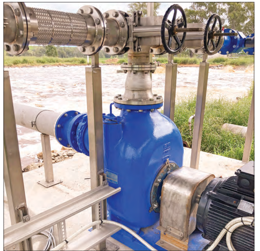
With more than 10 Gorman-Rupp T3 pumps at Bush's Proteins, the recent T10 addition "is doing a great job. They're pretty much bulletproof."
